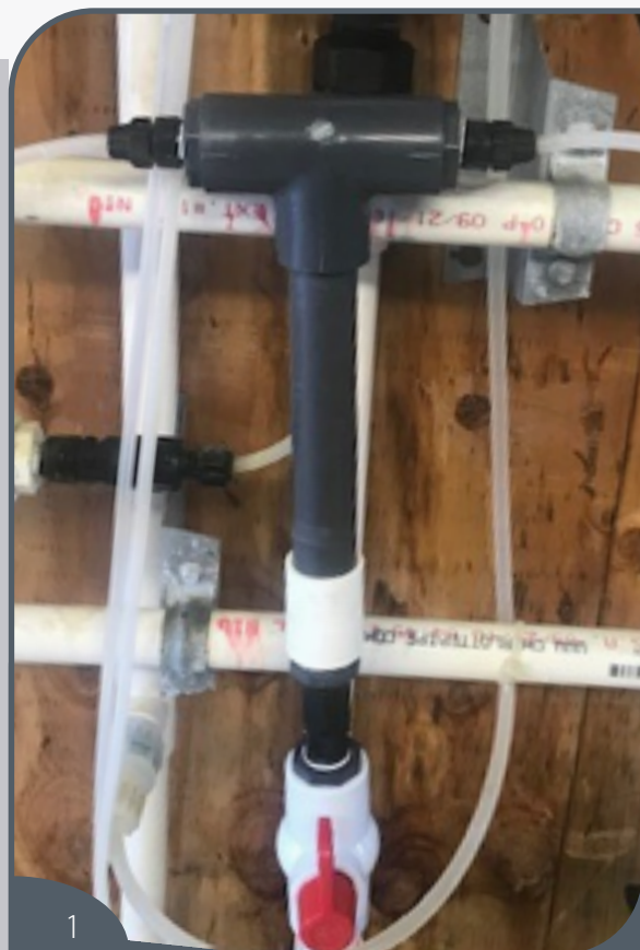
1 An in-line chamber provides improved reaction time for chlorine dioxide.
